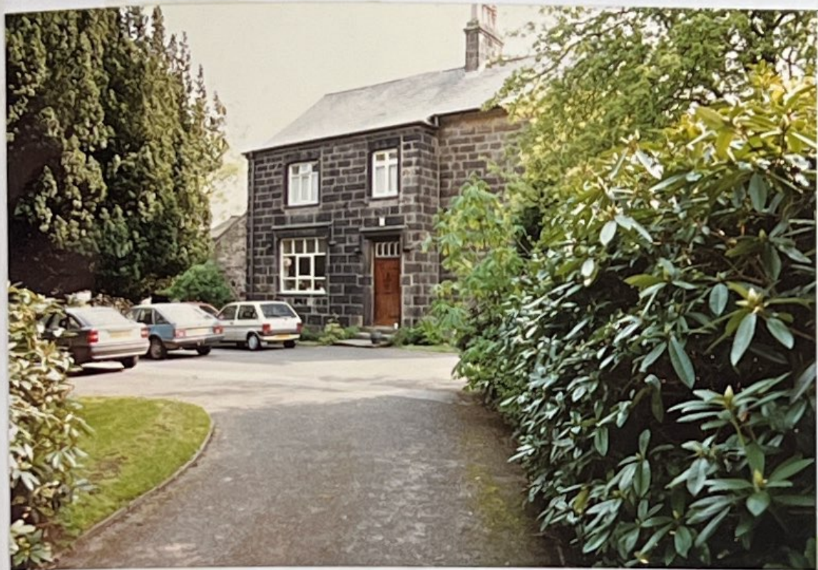
Front of the original vicarage. Note how the first step to the entrance has been worn away by the passage of feet over some 150 years.
